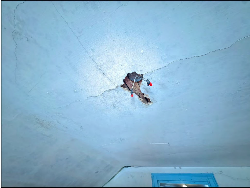
Plate 348. Electrical outlet on ceiling.
