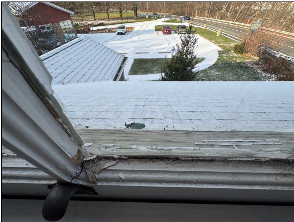
Plate 286. Detail of wood sash deterioration, failed glazing, chipped paint and overall weathering.
