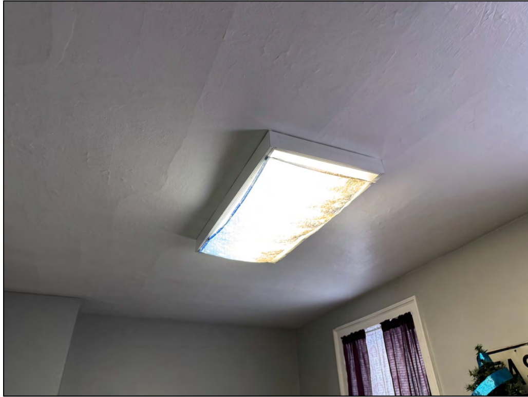
Plate 319. Note layers of uneven plaster on ceiling.
