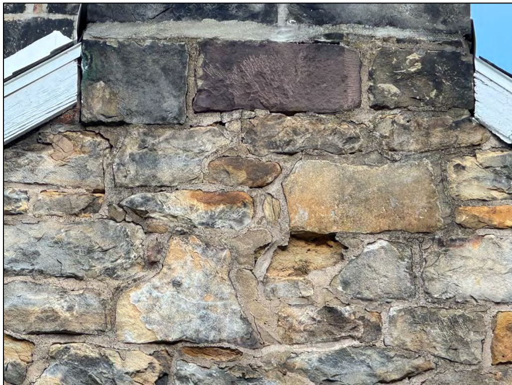
Plate 23. South Elevation, base of gable end chimney. Note the deteriorated stone and incompatible mortar.
