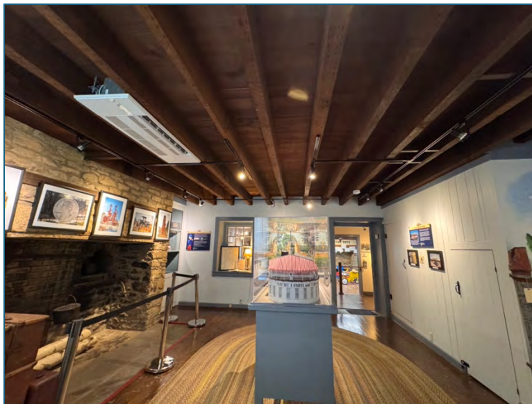
Photo 11. View of the HVAC system in the Ship room, facing west.
