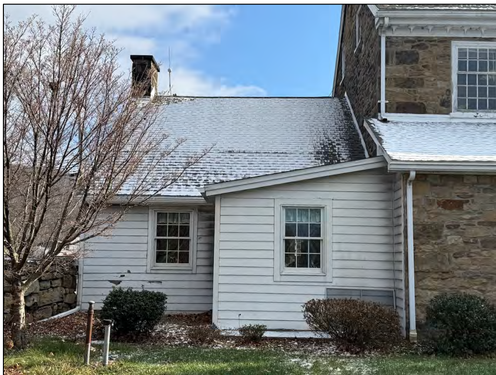
Plate 74. West elevation, facing east. Note the flaking paint and sediment on the walls.
