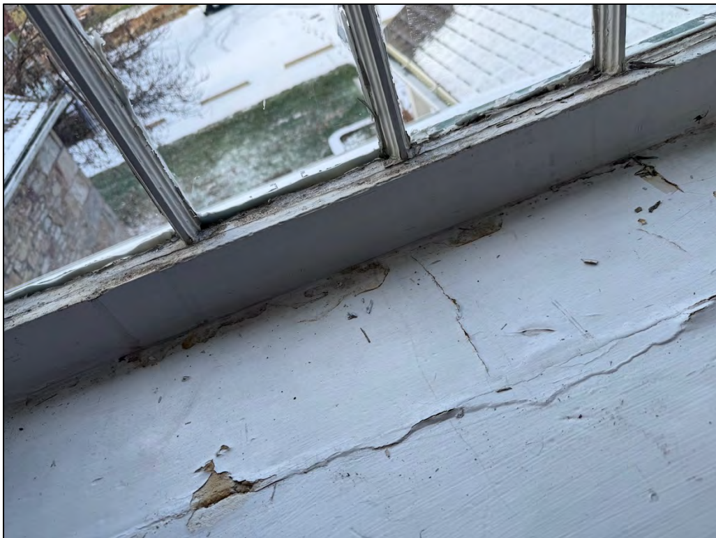
Plate 318. Detail of wood window and apron deterioration.
