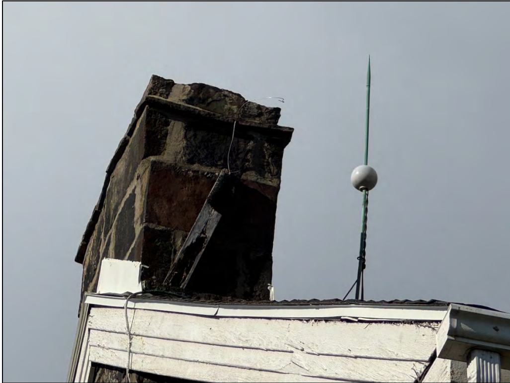
Plate 65. Chimney 3, facing west. There is no cap on the chimney.
