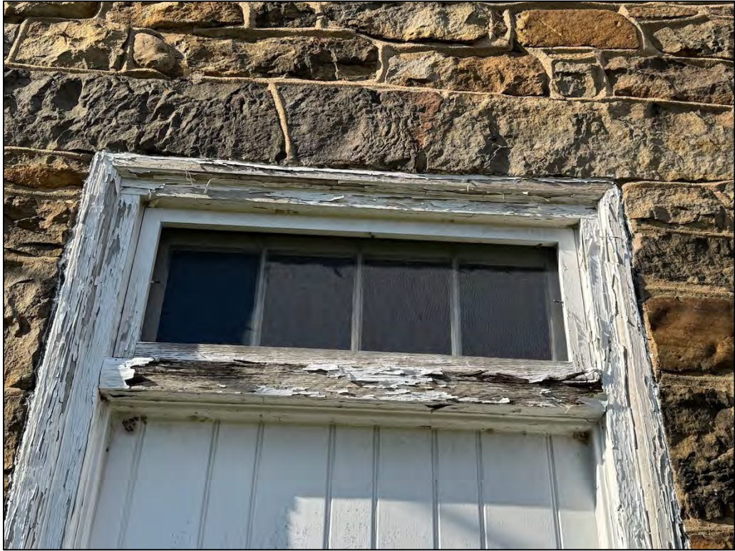
Plate 99. The transom on the west elevation. Note the screen frame in transom and deteriorated paint.
