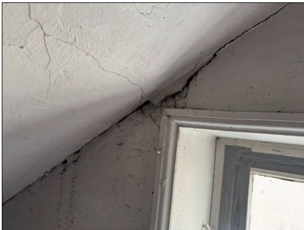
Plate 273. Room 13, facing north. Crack at ceiling/wall juncture.
