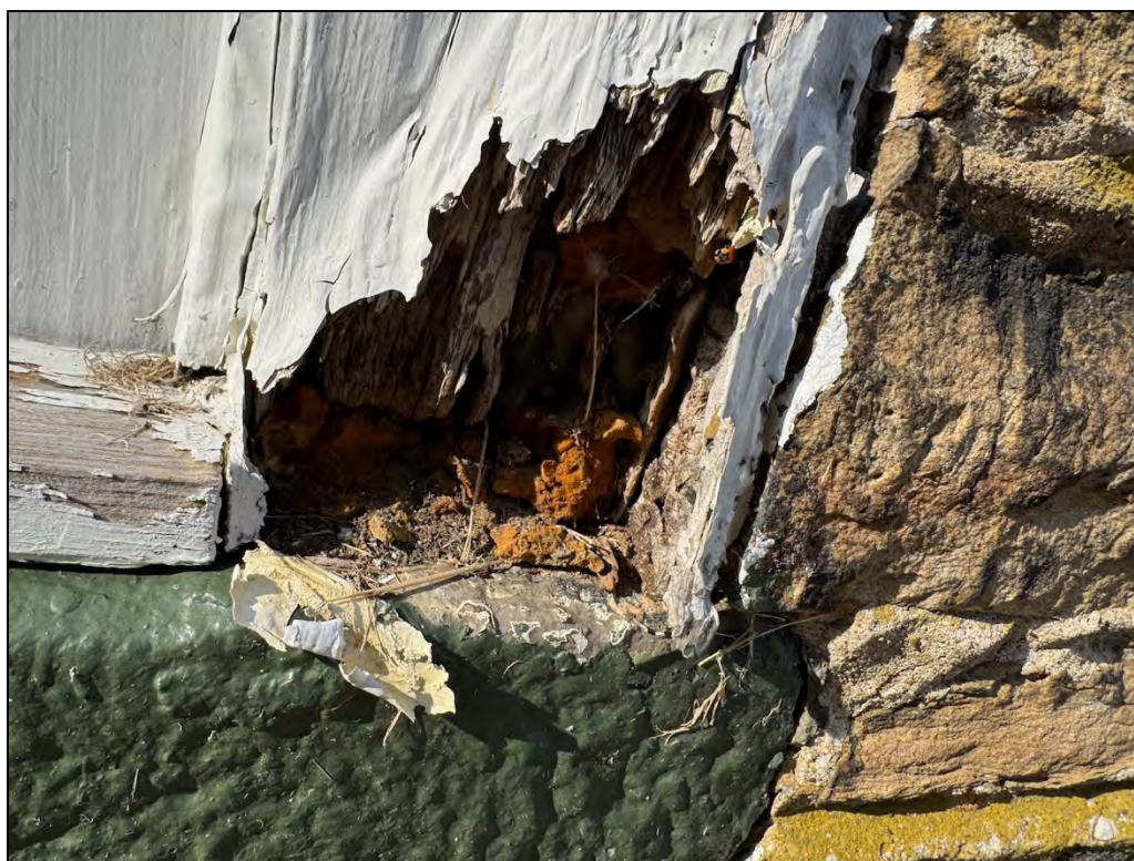
Plate 98. Lower right corner of front door. The hole was previously filled with foam which has been removed, (possibly by vermin).
