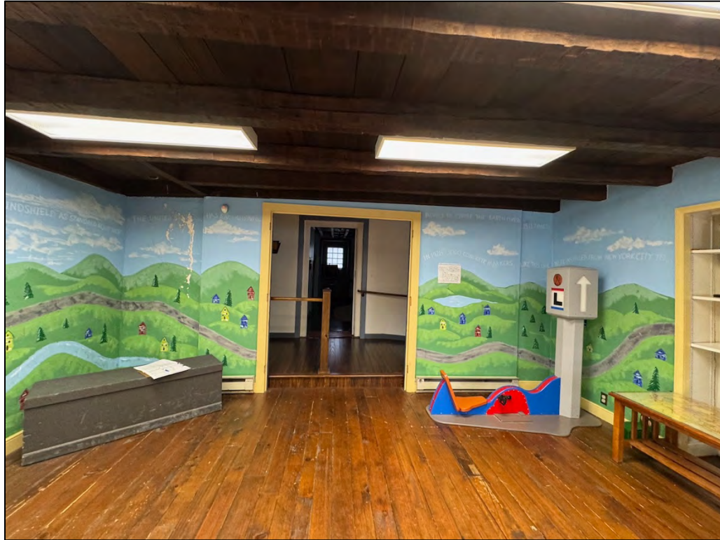
Plate 232. Tot Room, facing east. Note water damage to the left of the cased opening.
