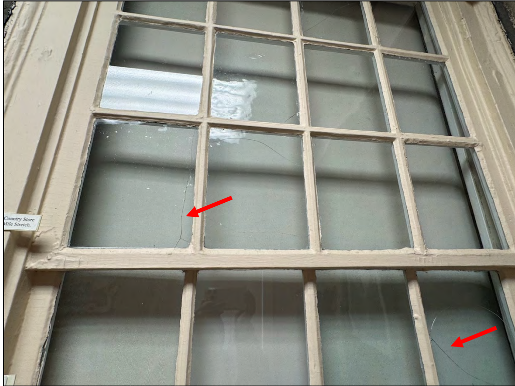
Plate 137. Typical cracked glass in window.
