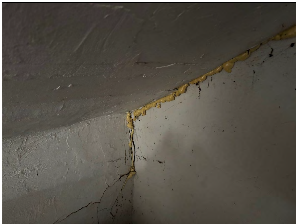
Plate 271. Room 13, facing southeast. Note crack infilled with spray foam and thick plaster.
