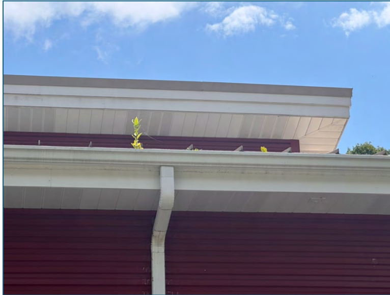
Photo 2. Gutter on west elevation clogged with debris.
