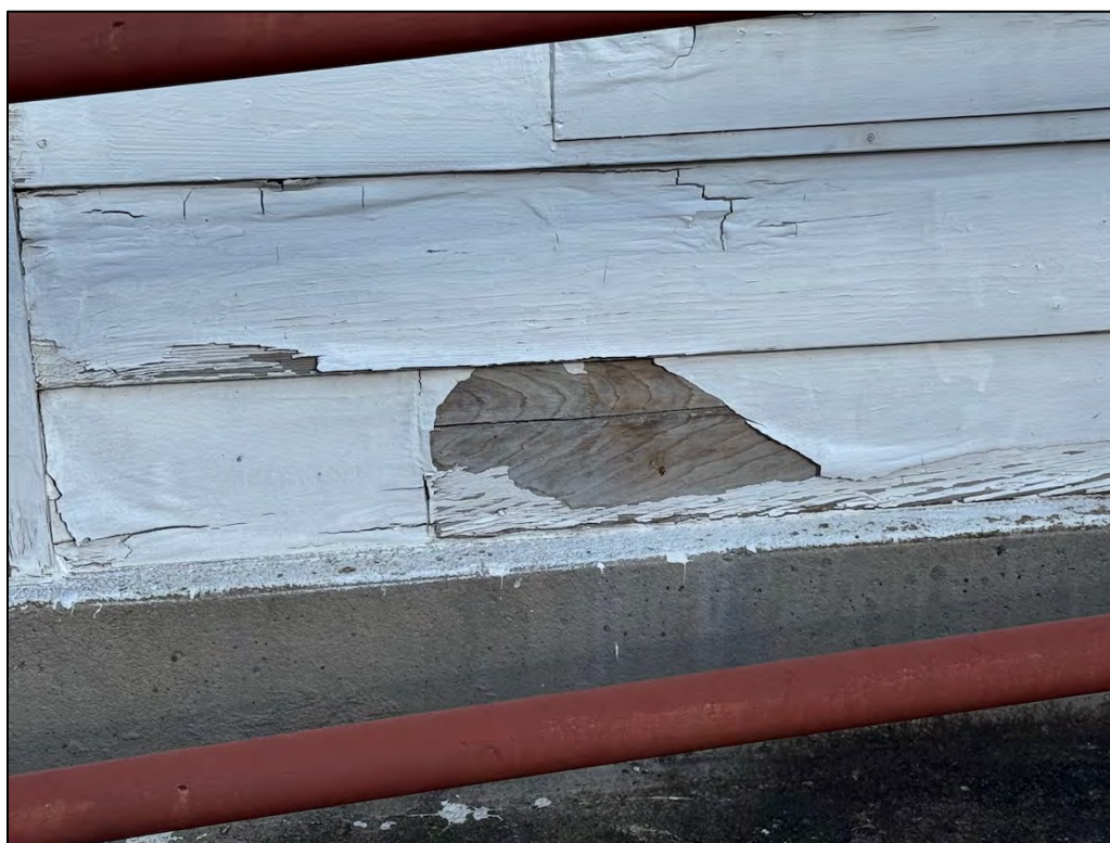
Plate 81. Detail of water damaged siding.
