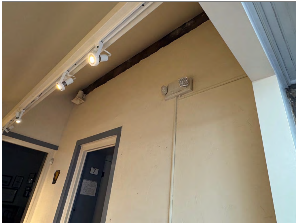
Plate 250. Ceiling in hallway outside of Ship Room, note exposed wood.
