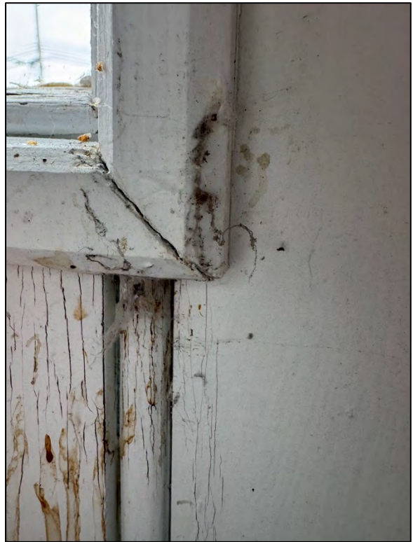
Plate 161. Note deterioration in door, including insect debris and staining. Facing east.
