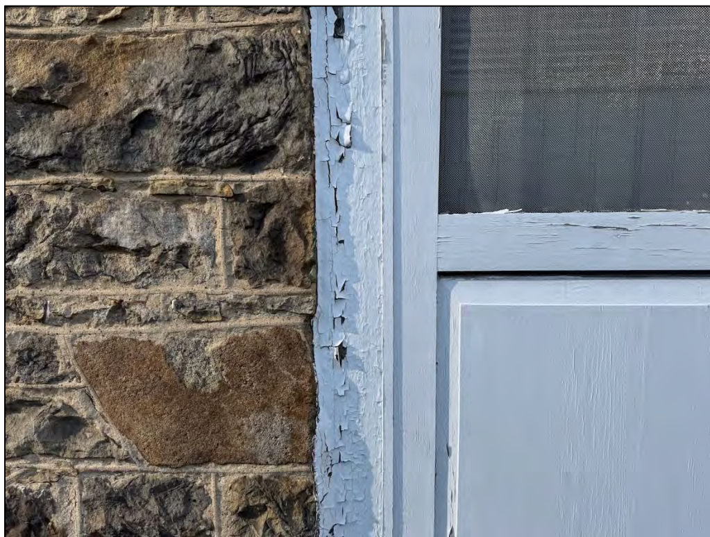
Plate 105. Wood frame of screen door with flaked paint.
