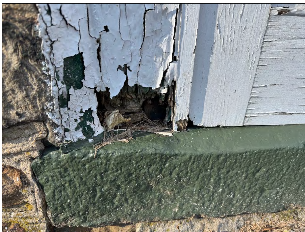
Plate 104. Detail of lower left of door. Note deteriorated wood and flaked paint.
