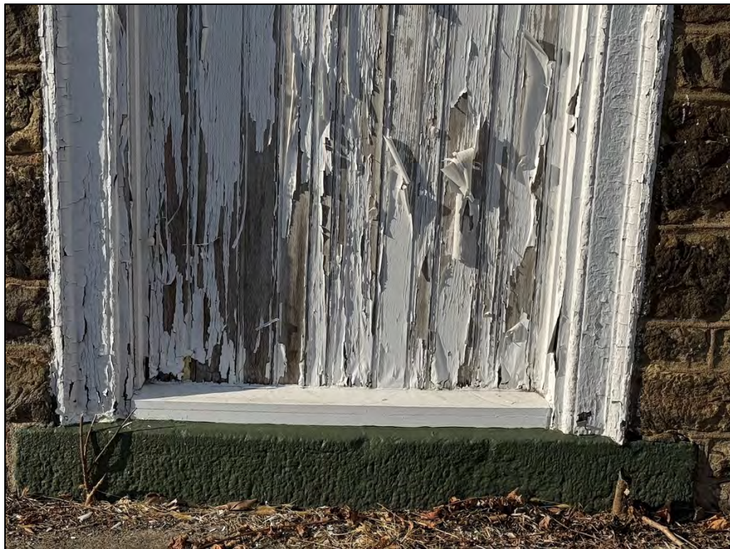
Plate 86. Base of door, deteriorated wood and flaking paint.
