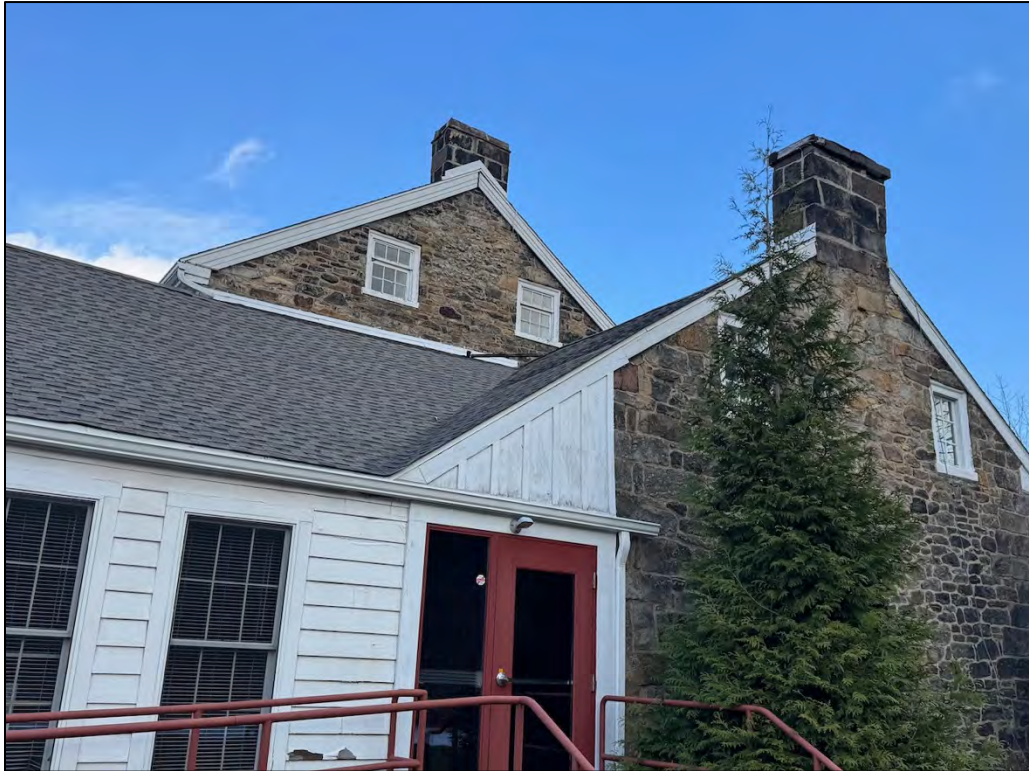
Plate 29. South elevation. Note the foliage which is too close to the building.
