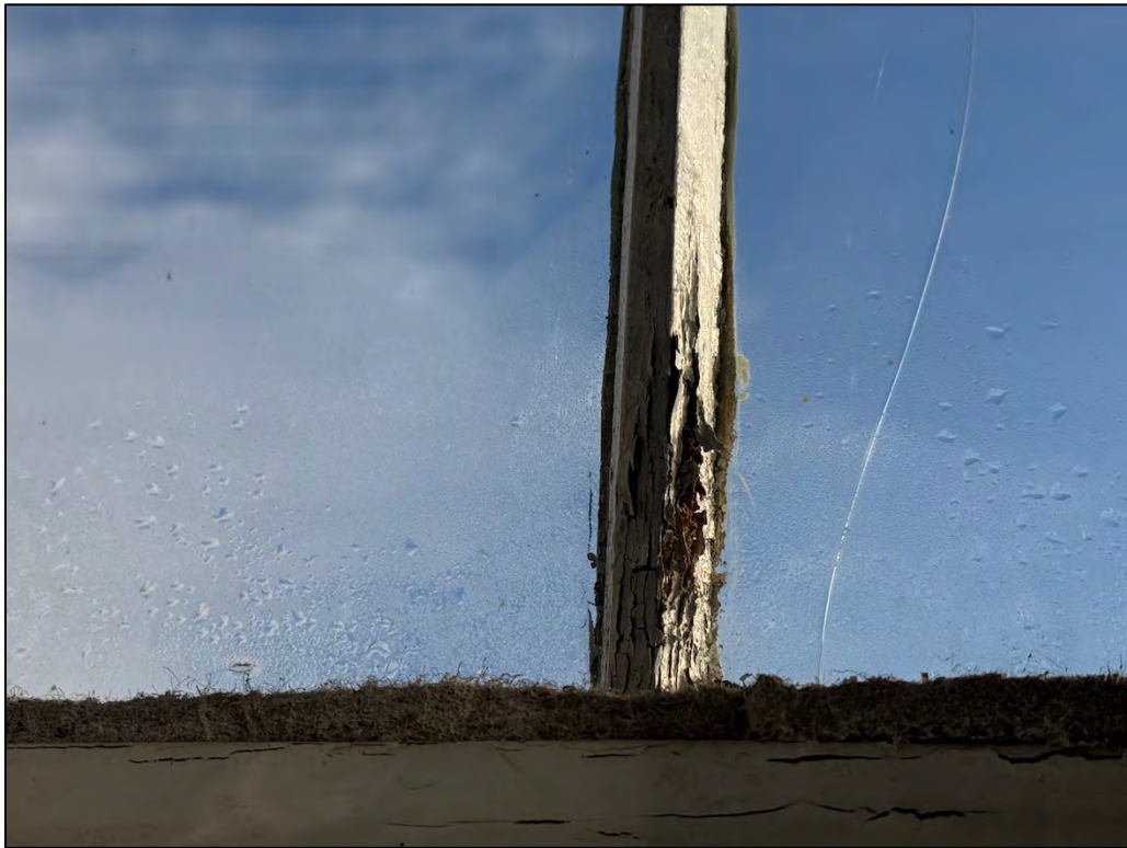
Plate 298. Deterioration, lack of glazing, moisture on interior of window.
