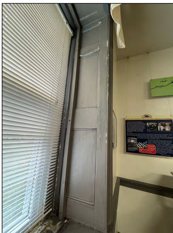
Plate 213. Deteriorated shutter on window 1-16, facing southeast.
