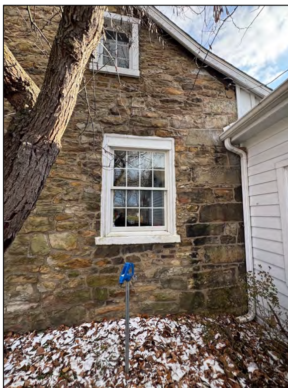
Plate 33. West Elevation, mortar previously repointed, some organic staining
