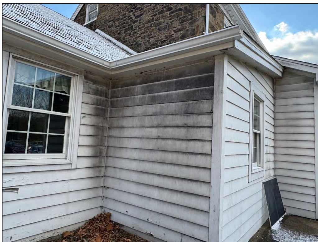
Plate 78. North side of the addition, note the peeling paint and sediment.
