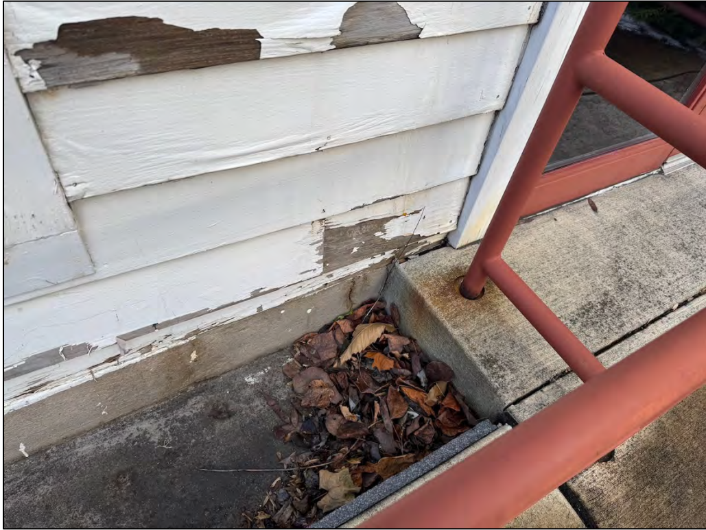
Plate 82. Additional water damage on east side of the south elevation.
