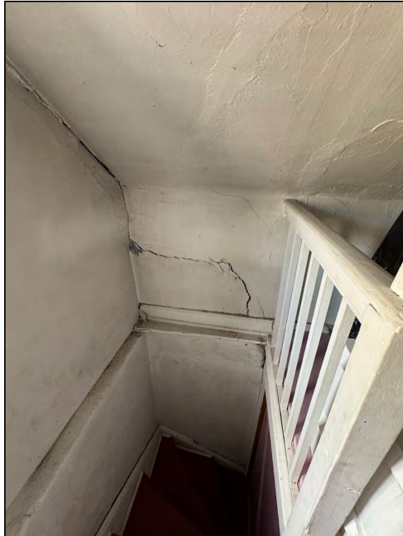
Plate 270. Room 13, facing east. Note the major crack in the wall.
