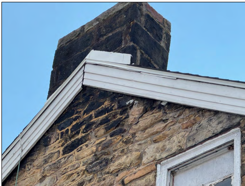
Plate 36. North elevation, note the staining of the stone and incompatible mortar
