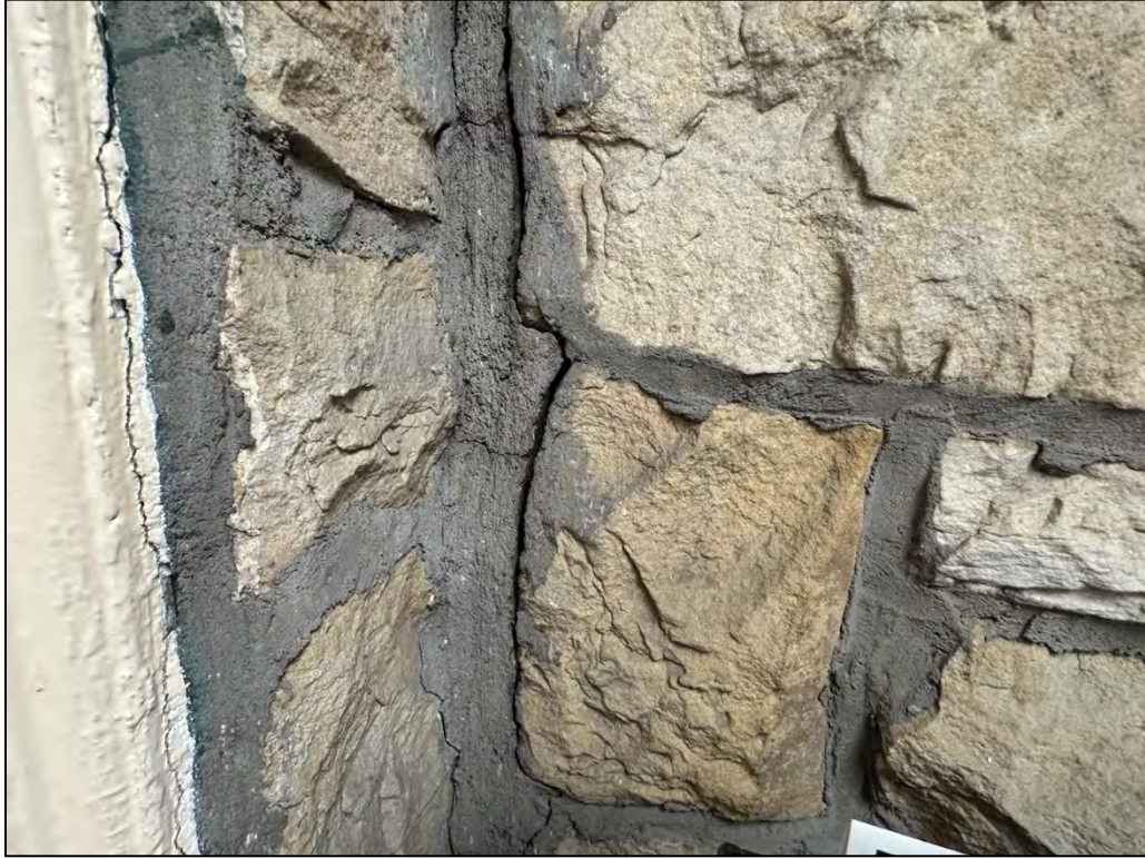
Plate 139. Cracked mortar, facing southeast.
