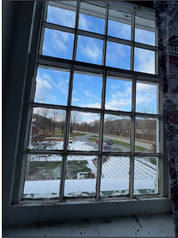
Plate 317. Wood window, facing west. Note cracked sill.
