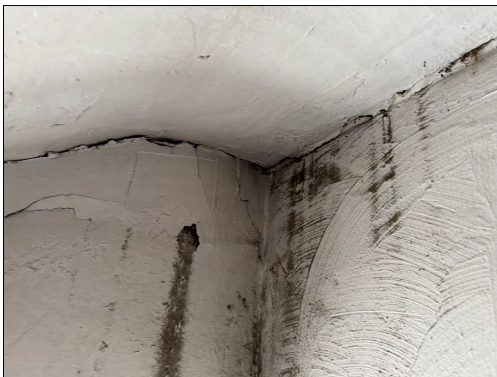
Plate 274. Room 13, facing east. Note crack at wall/ceiling juncture.
