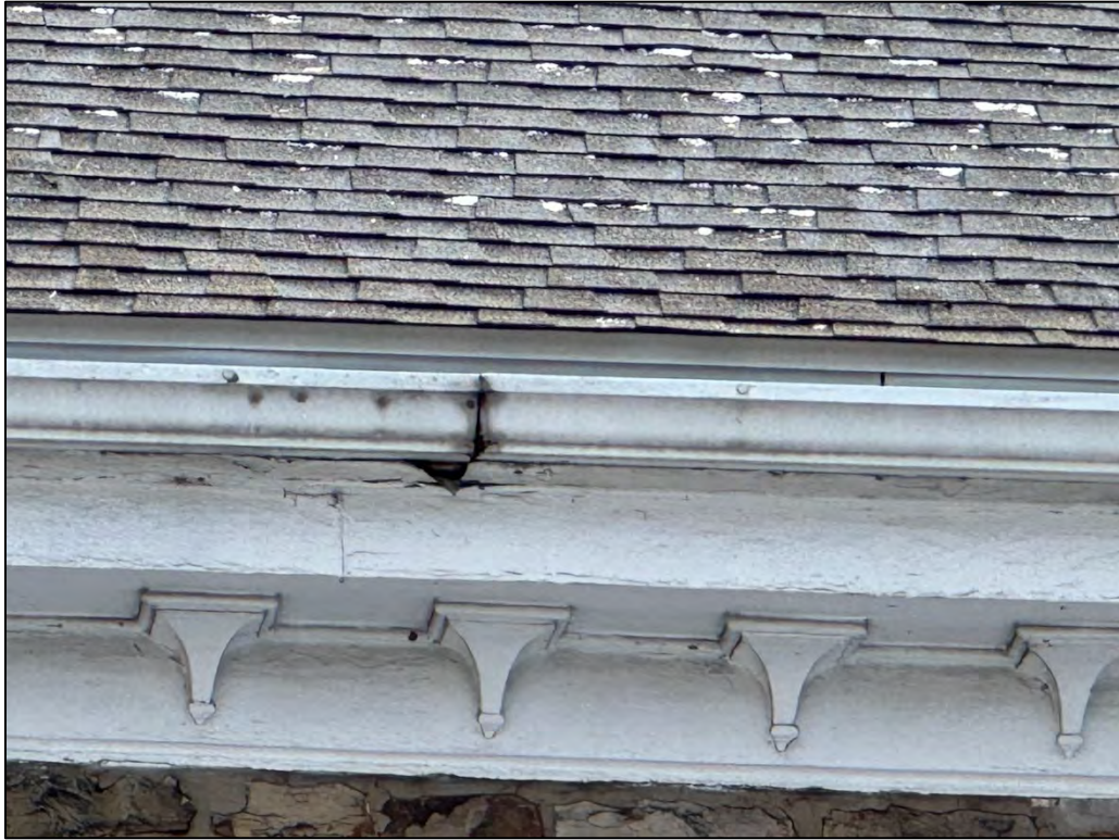
Plate 47. Overall, the gutters on the main building are damaged with broken joints, holes and deterioration.
