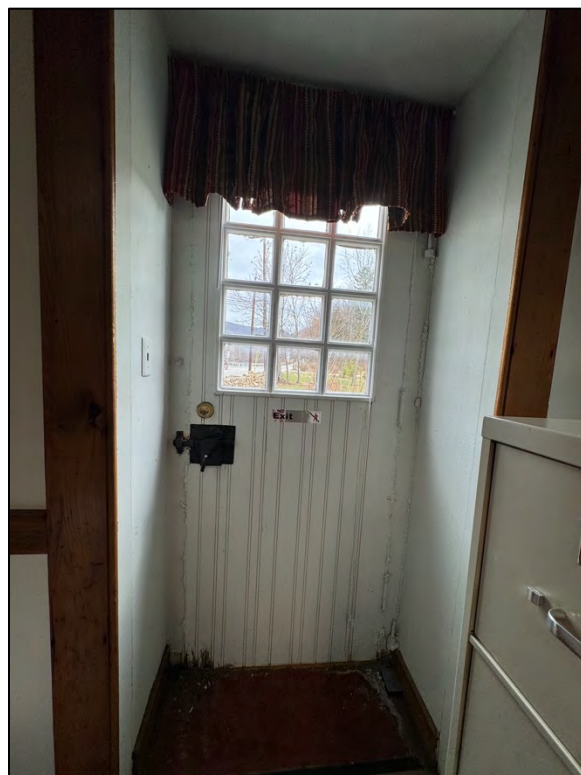
Plate 156. Detail of the door, facing east. Note deterioration on the lower portion of the door.
