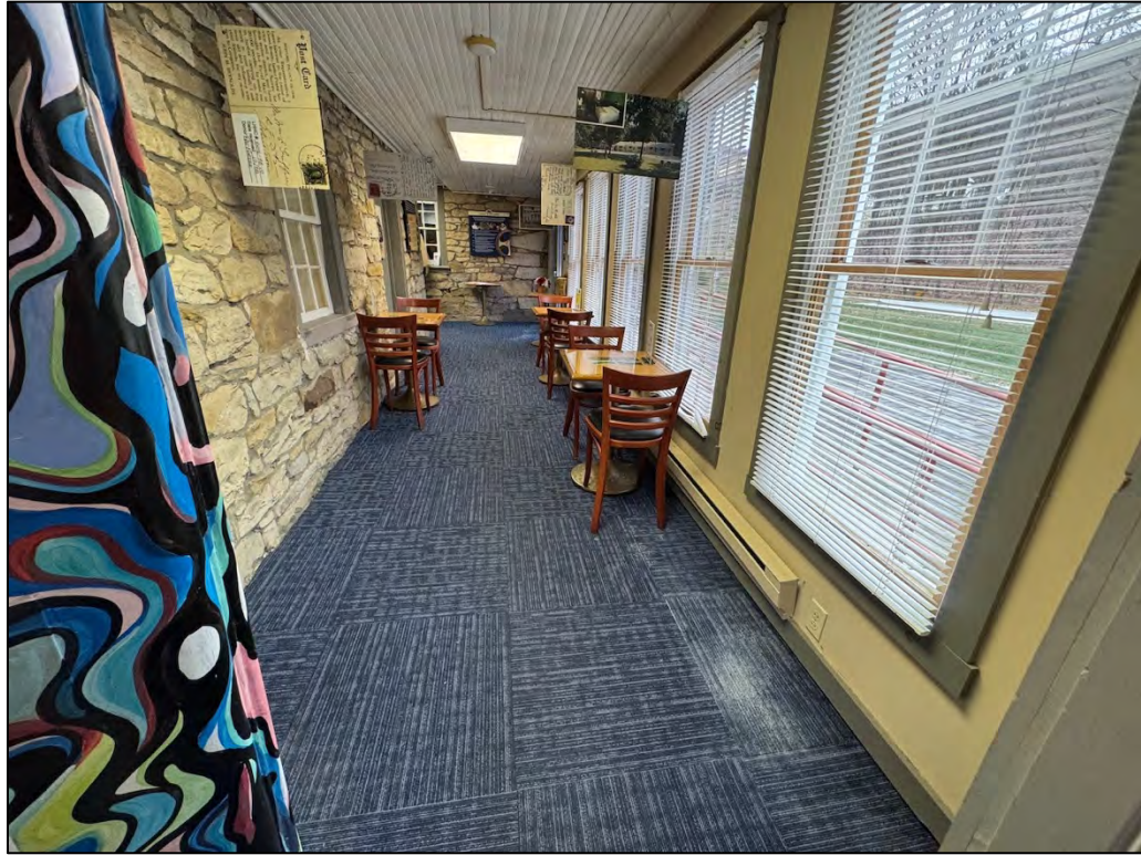
Plate 255. Postcard Corridor, facing east. Note efflorescence on carpet.
