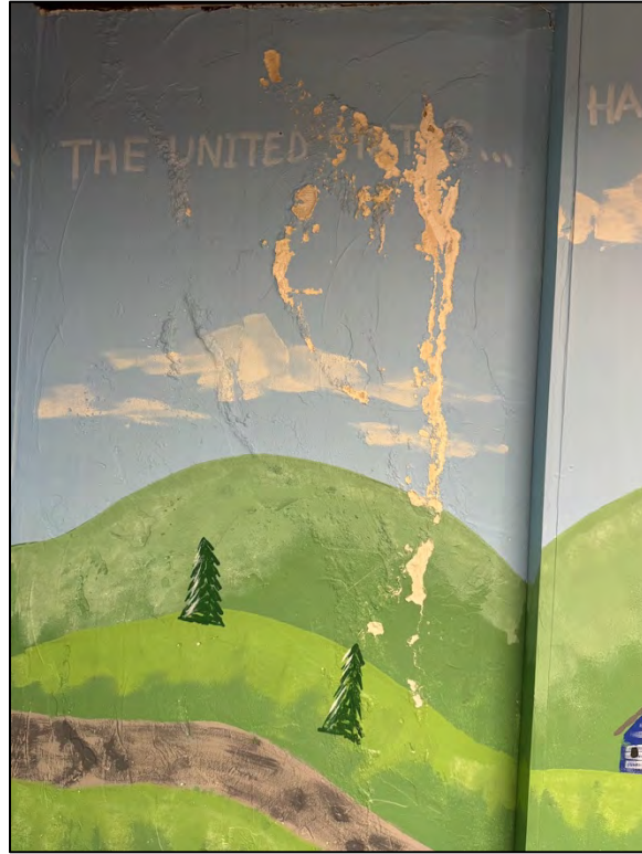
Plate 246. Deterioration due to moisture on plaster wall, facing east.
