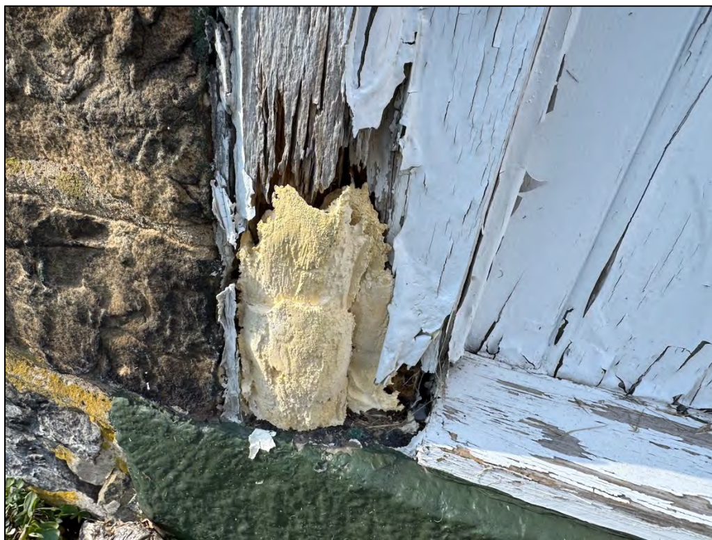
Plate 97. Lower left corner of the front door. Note the deteriorated wood and flaked paint.
