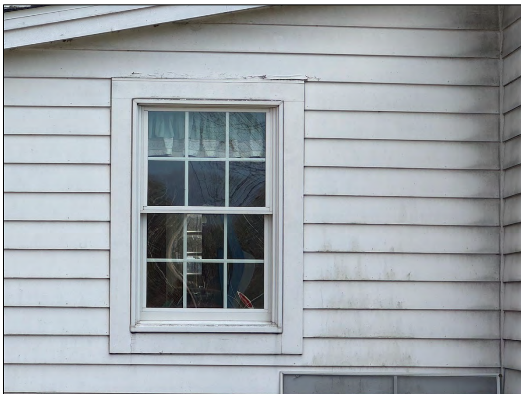
Plate 75. West elevation, facing east. Note the flaking paint at the top of the window.
