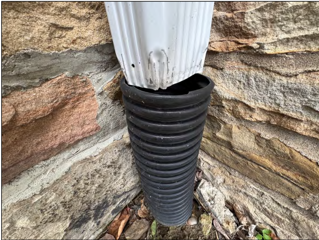
Plate 44. Detail of downspout not directly connecting with drain. Splash back can erode surrounding stone more quickly.
