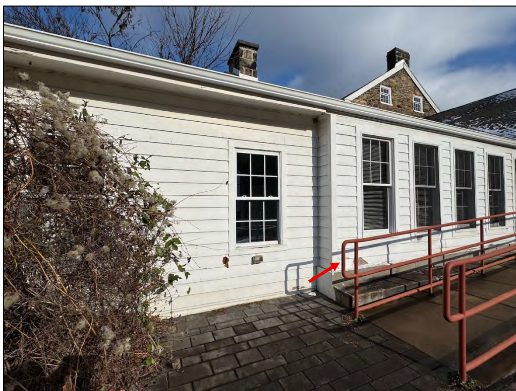
Plate 79. South elevation, facing north. Note peeling paint.
