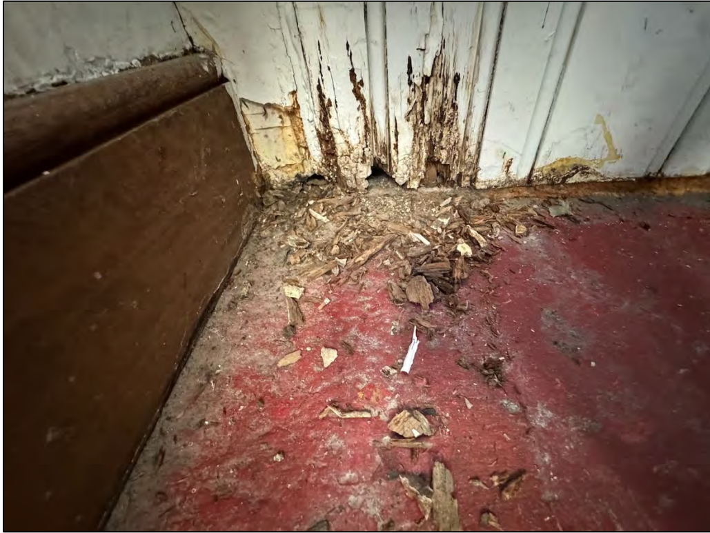
Plate 157. Detail of the deterioration of the door, lower left corner, facing east.
