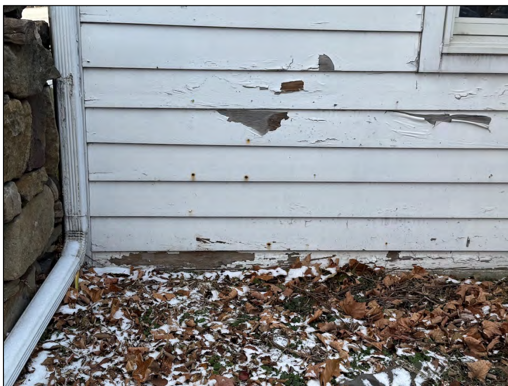
Plate 77. Deteriorated paint on siding, west elevation.
