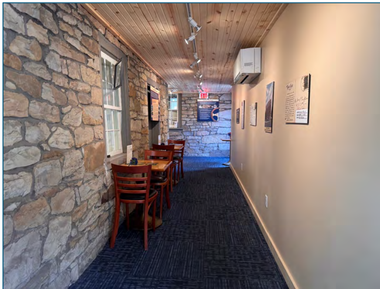
Photo 9. The HVAC system is placed on the exterior wall in the Postcard Corridor.
