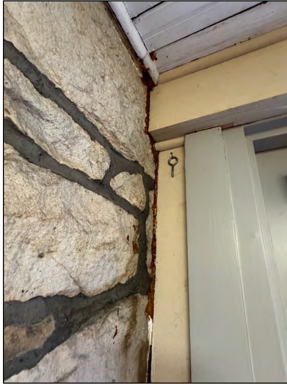
Plate 261. Spray foam in between exit door and stone wall, facing southwest.
