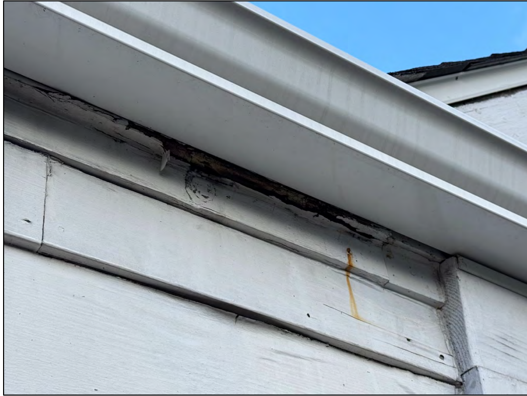
Plate 84. Deteriorated eaves may indicate a faulty gutter.
