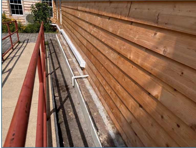
Photo 6. South elevation, facing west. Note the wall is slightly pulled in, away from the edge of the building. The drain line empties onto the concrete below.
