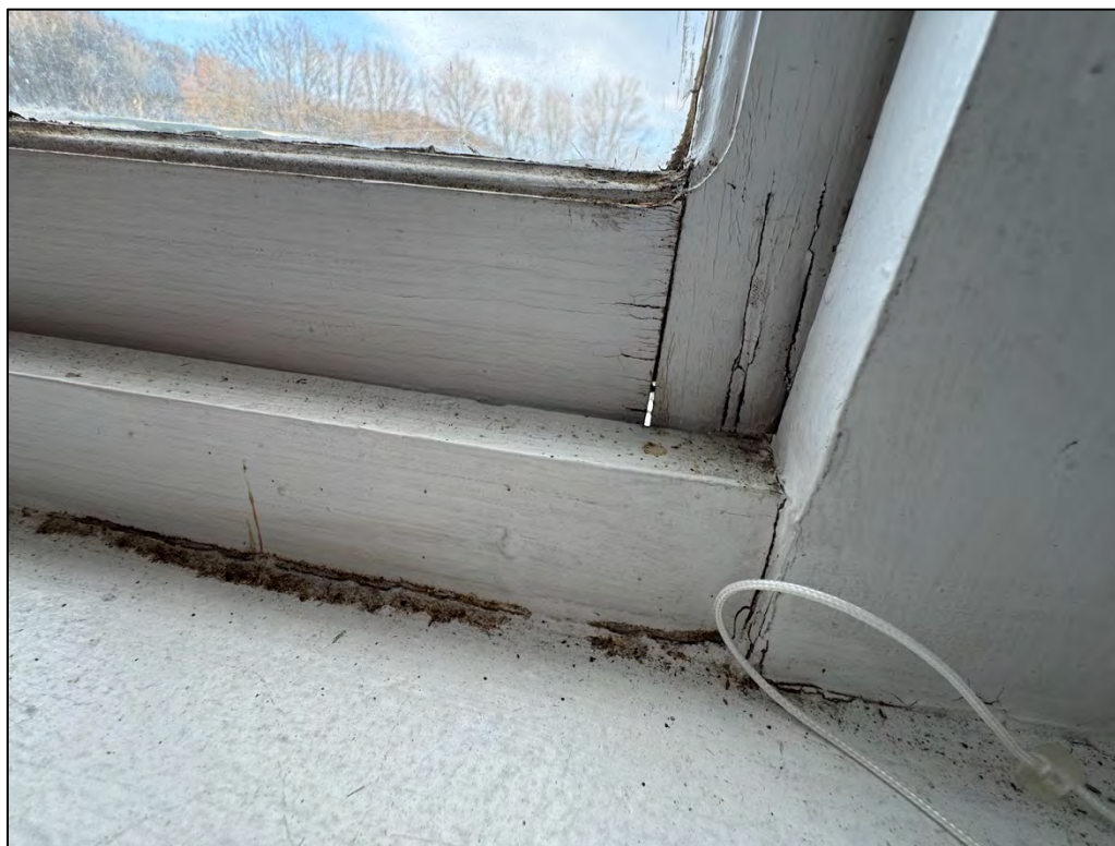
Plate 287. Room 14, Stile and rail separation; staining indicates moisture infiltration and insect activity.
