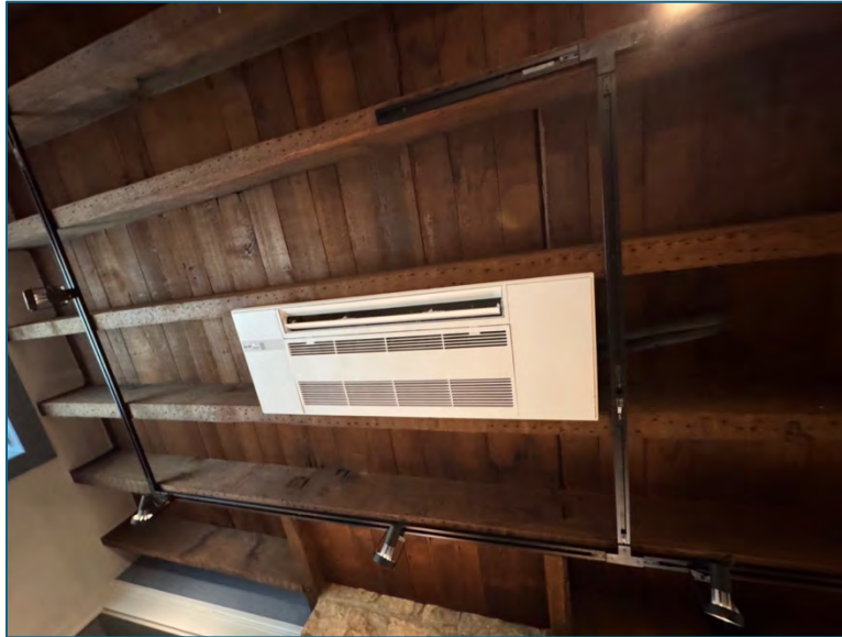
Photo 12. Detail of the HVAC system in the Ship room.
