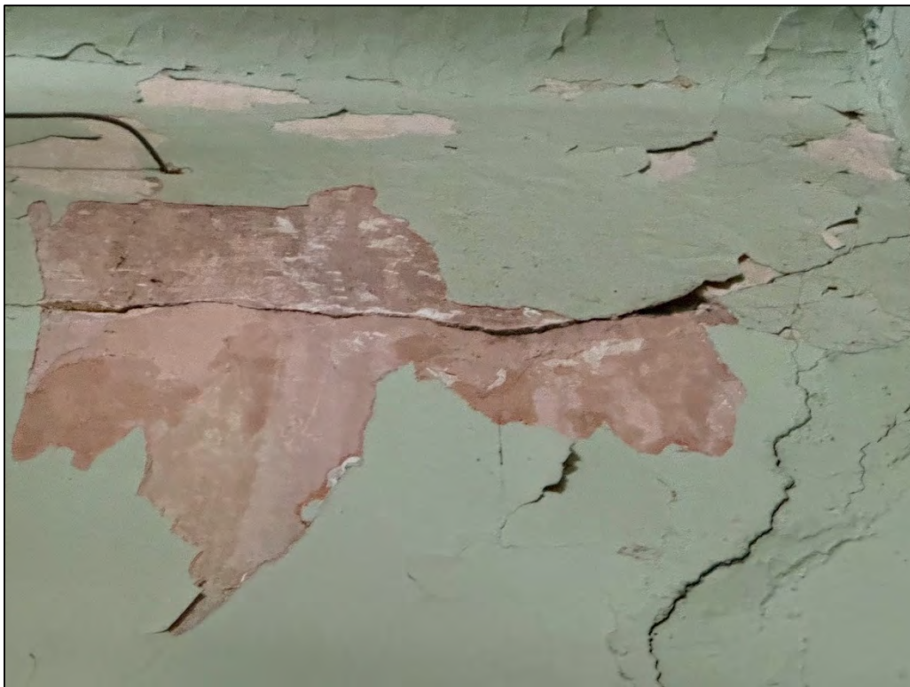
Plate 332. Detail of plaster damage and repair.
