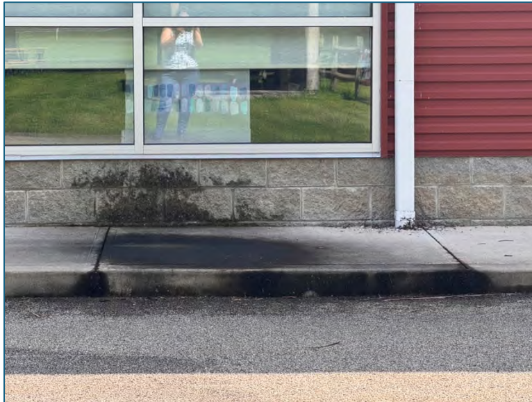
Photo 1. Organic staining on the sidewalk. Note the bird droppings at the base of the downspout.
