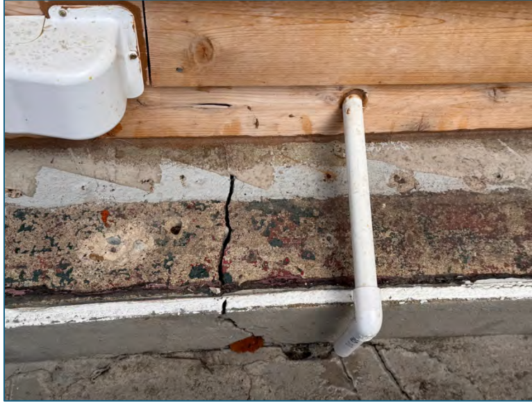
Photo 8. Note the condition of the concrete wall. The cracks are allowing water to infiltrate the masonry and should be addressed.
