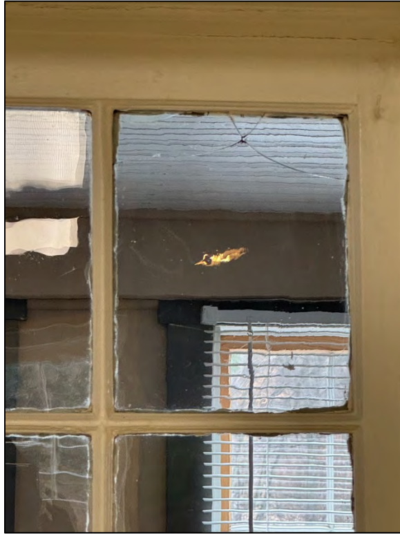
Plate 240. Example of cracked glass in upper sash, facing south.
