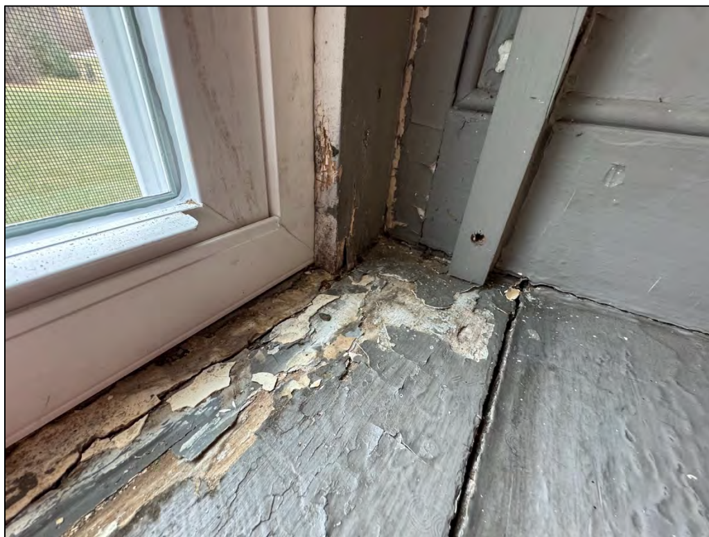
Plate 208. Window 1-16, detail of water damage, facing southeast.
