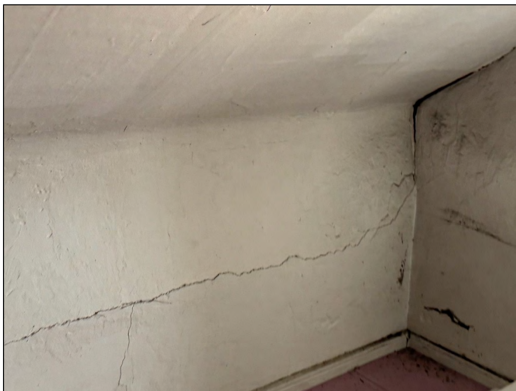
Plate 277. Room 13, detail of crack, facing west.
