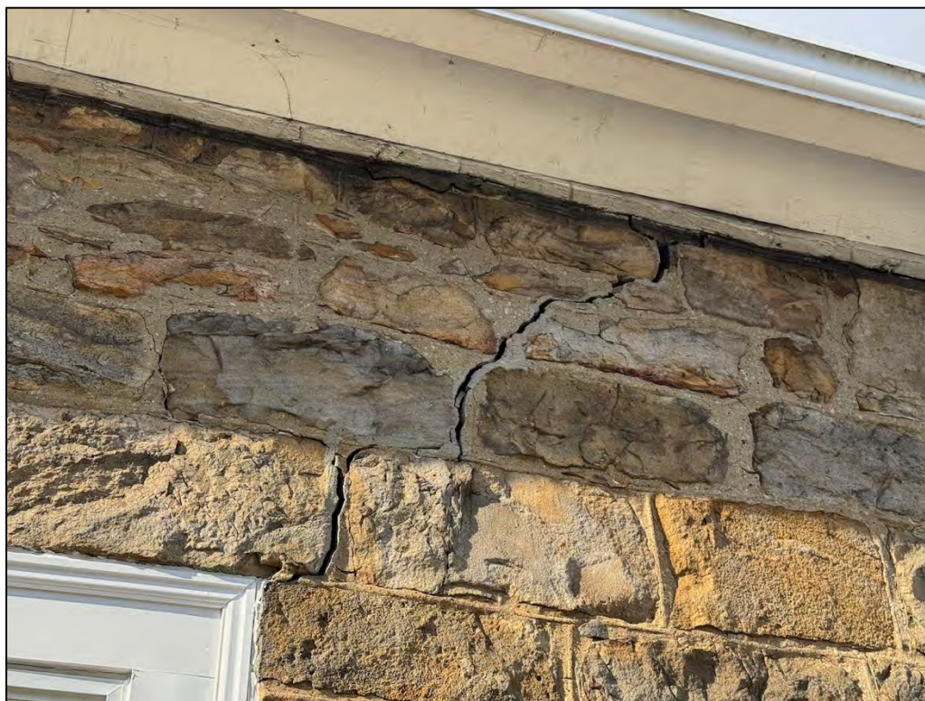
Plate 24. Stairstep crack in northern wing, east elevation.
