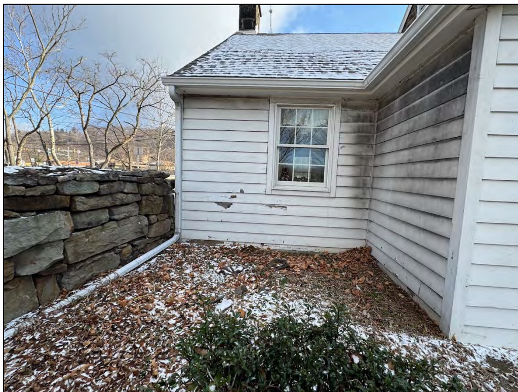
Plate 76. West elevation, facing east. Note the flaking paint and sediment.
