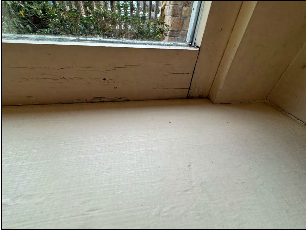
Plate 141. Deterioration of the window, west elevation.
