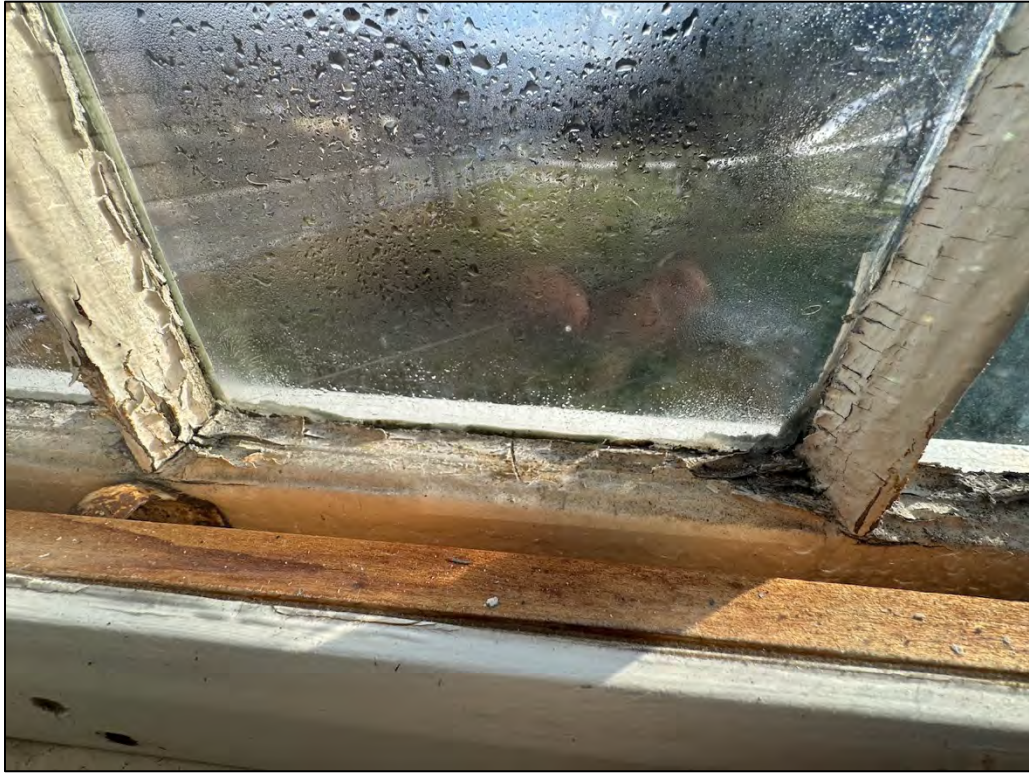
Plate 297. Detail of deterioration caused by condensation, insects and sunlight, facing east.
