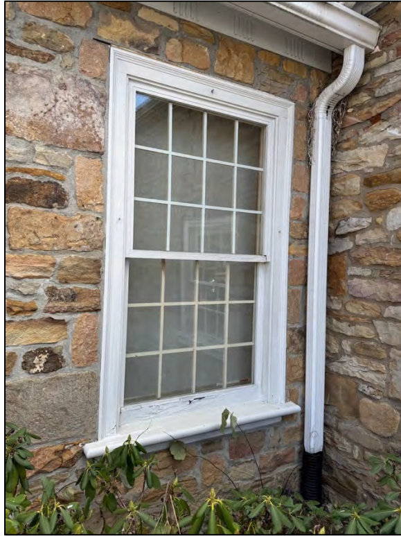
Plate 43. West elevation (enclosed porch). Typical gutter and downspout. Note the bird nest against the house.
