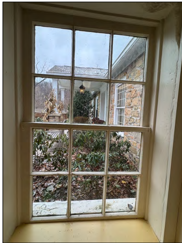
Plate 235. Wood window, facing north. Note the scratch in the glass.
