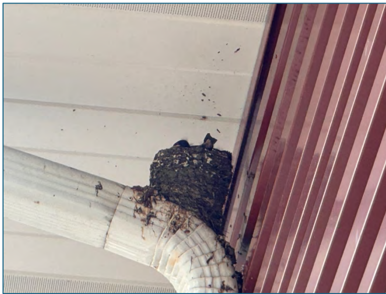
Photo 3. Evidence of bird's nest on downspout.
