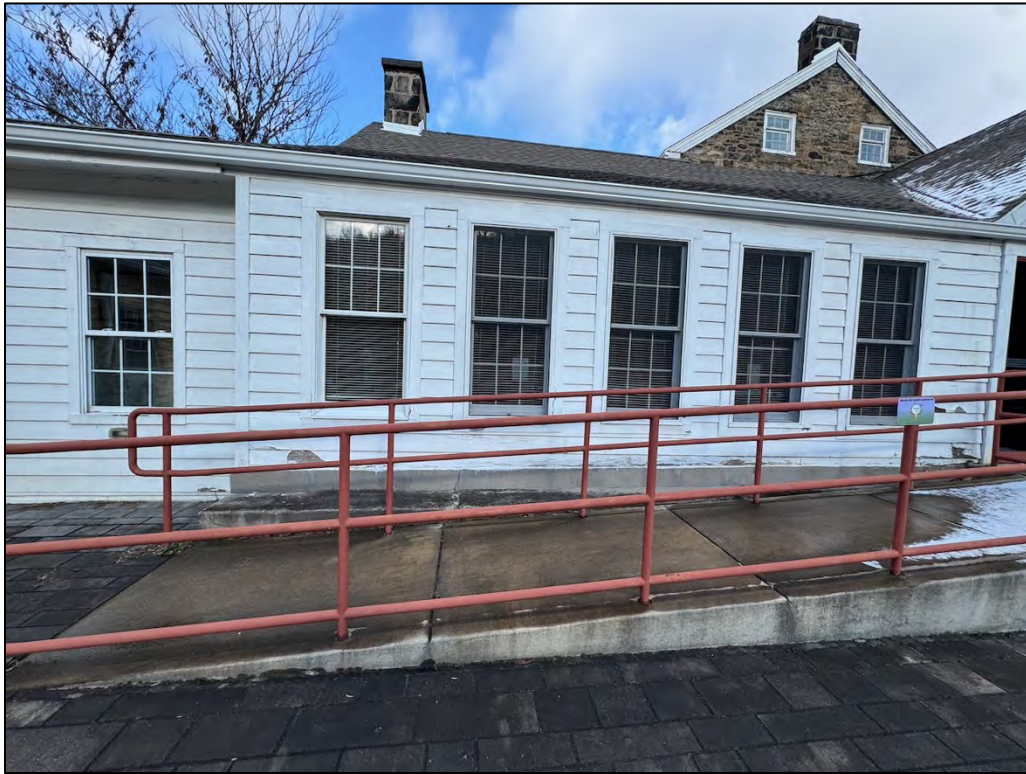
Plate 51. Existing gutter on enclosed porch. Water damage is affecting the nearby siding. [See 2026 updated in Appendix].
