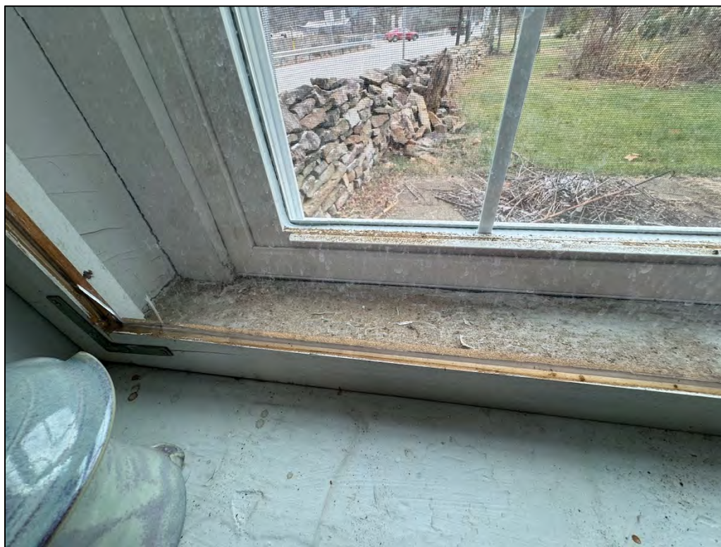
Plate 155. Room 4, Detail of the window debris, facing east. Note the broken wood storm window, separation between the window frame and the wall and the insect staining.
