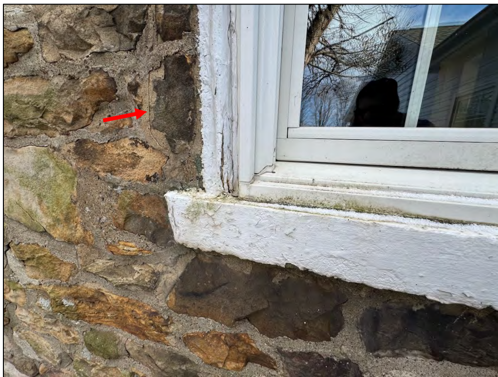
Plate 34. Detail of crack north side of window
