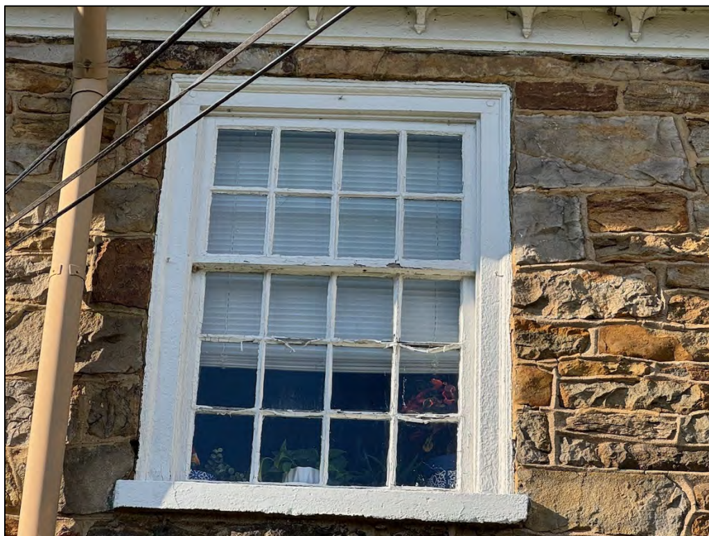
Plate 118. Replacement wood window, east elevation (W2-9). Note the deterioration of the muntins and glazing.
