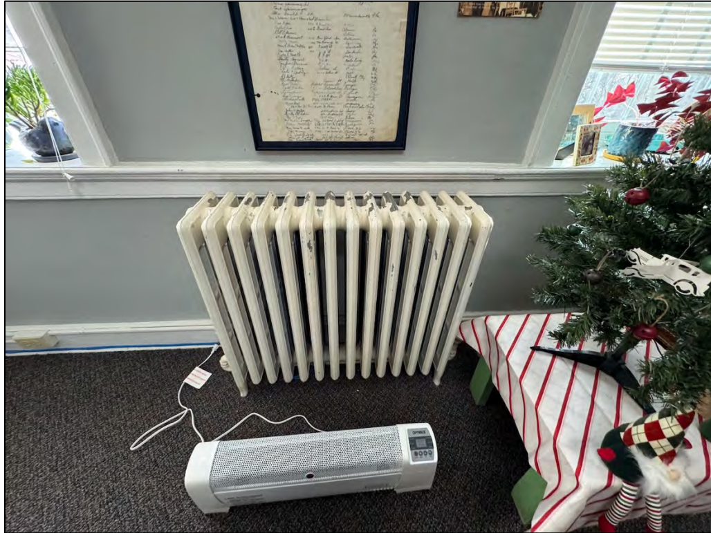
Plate 308. Dual radiators, facing east.
