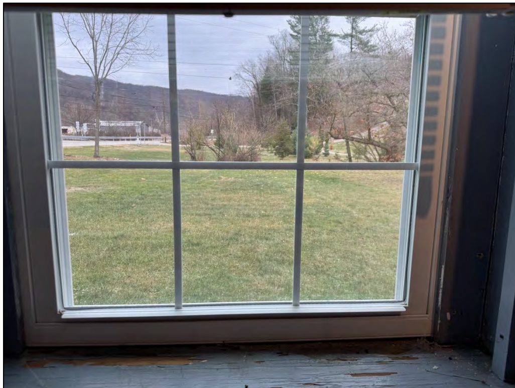
Plate 224. Replacement window in the Ship Room. Note the water damage to the sill and frame, facing east.
