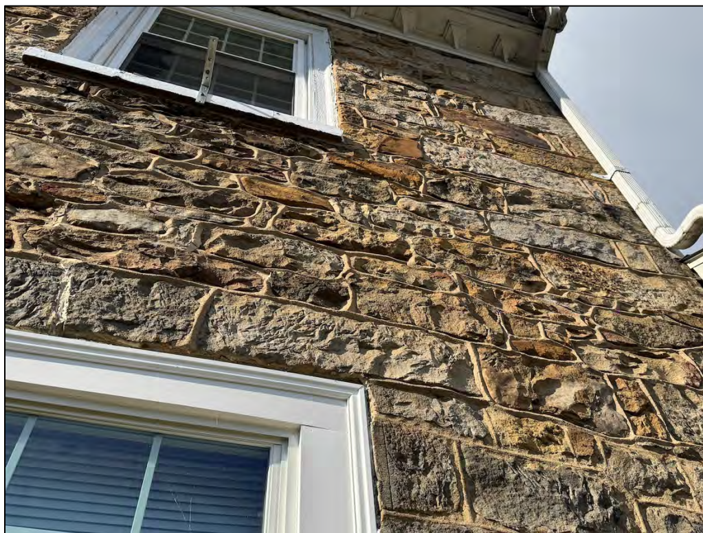
Plate 26. Angled view, east elevation, revealing differing weathering pattern of mortar and stone.
