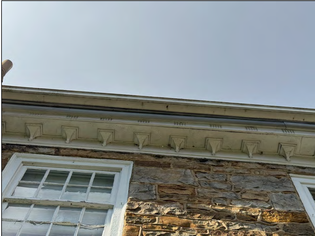
Plate 54. Detail of rust spots and holes in the gutter, east elevation.
