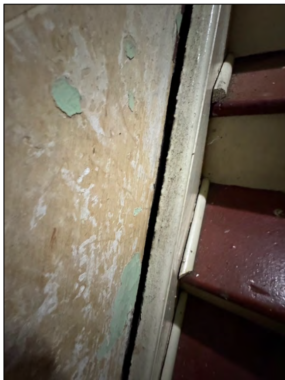
Plate 334. Stairs separating from the wall.
