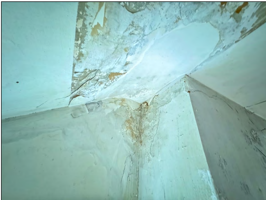
Plate 351. Plaster deteriorated walls facing south.
