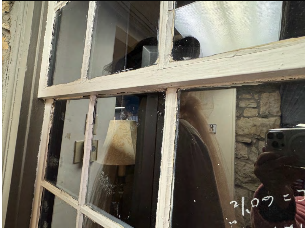
Plate 228. Typical condition of wood window, from hallway looking into Ship Room, facing northeast.
