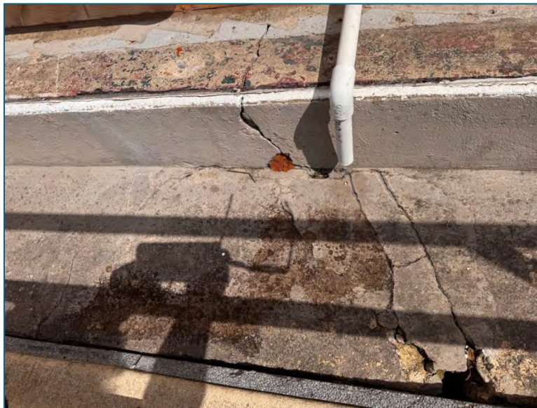
Photo 7. The drain line is emptying into a concrete basin. This has the potential to cause freeze-thaw deterioration of the concrete.
