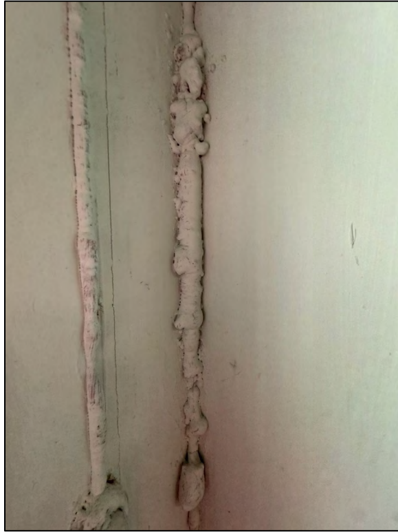
Plate 159. Painted spray foam residue, facing east.
