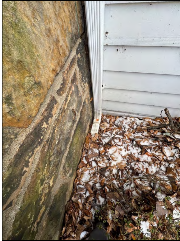
Plate 45. Need to ensure all downspouts are directed away from the foundation.
