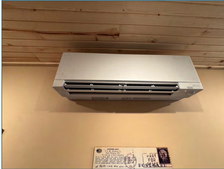
Photo 10. Detail of the HVAC system in the Postcard Corridor.
