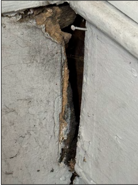
Plate 279. Room 13, large crack in wall, facing east.
