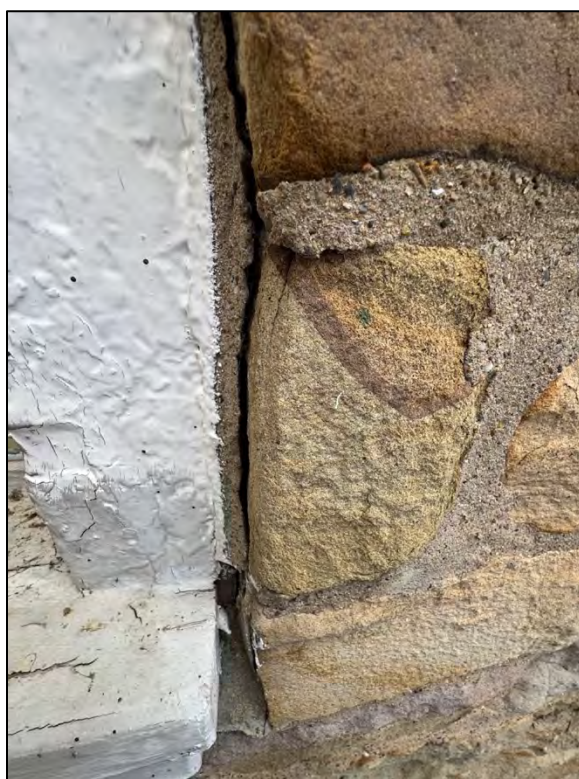
Plate 35. West side of window, north elevation of historic tavern/tot room. Note the space between the mortar and stone.
