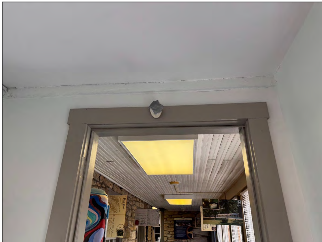
Plate 264. Detail view of ceiling wall connection, moisture damage, facing east.
