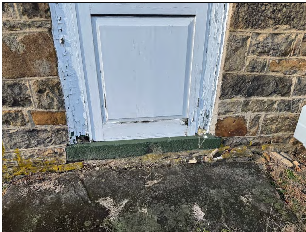
Plate 103. Deteriorated base of door.
