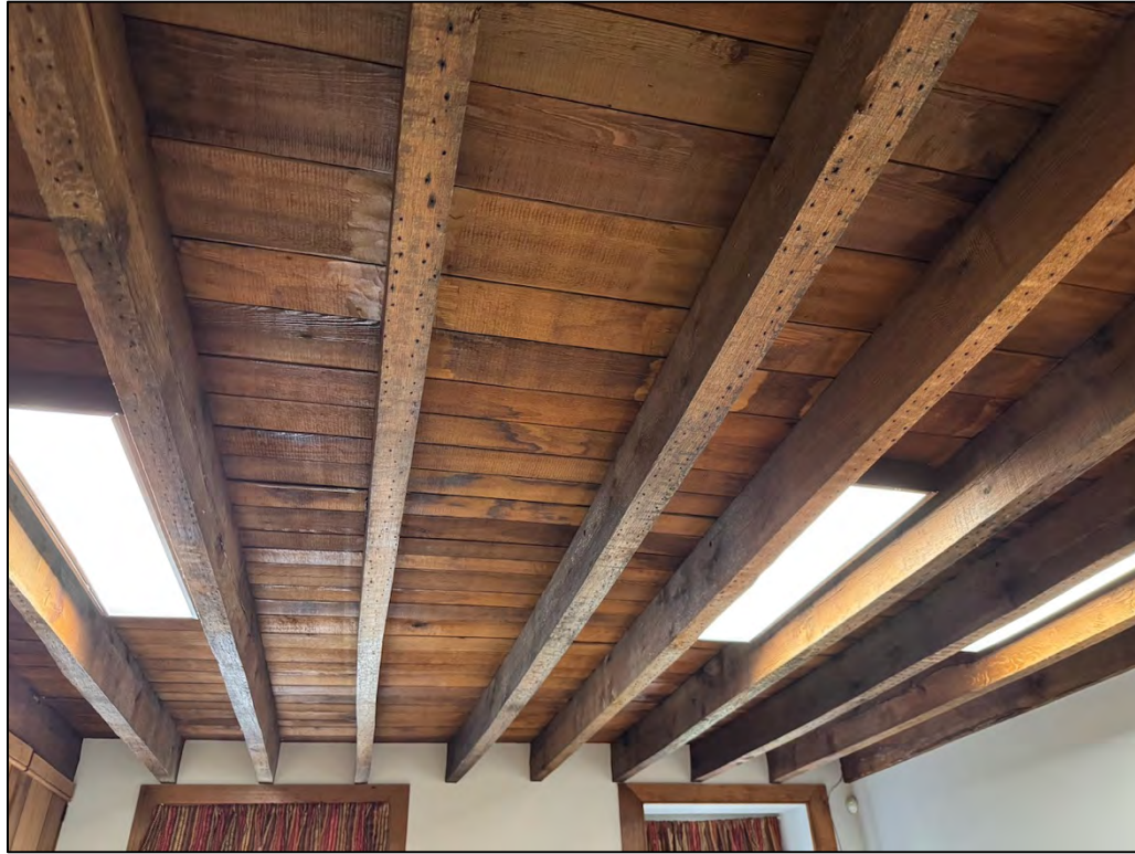
Plate 162. Detail of ceiling with nail holes, facing east.
