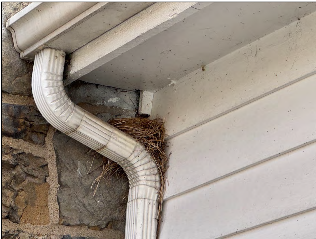
Plate 46. Several downspouts provide structural support for bird nests.
