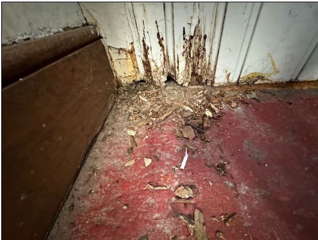
Plate 90. Bottom left corner (northernmost) of door. Note the deterioration of wood from moisture and insect activity.
