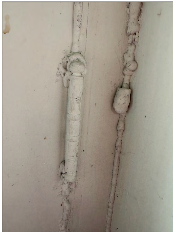
Plate 94. Painted hardware and painted insulation near door
