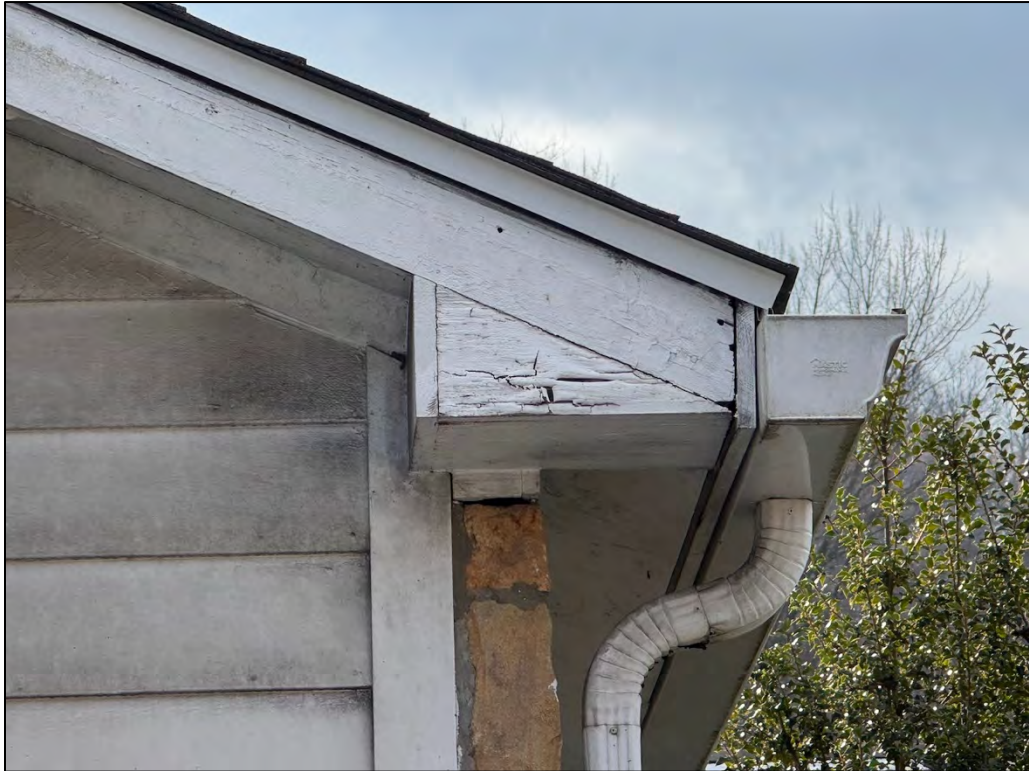
Plate 48. Typical connection of gutter and downspout. Deteriorated paint on fascia.
