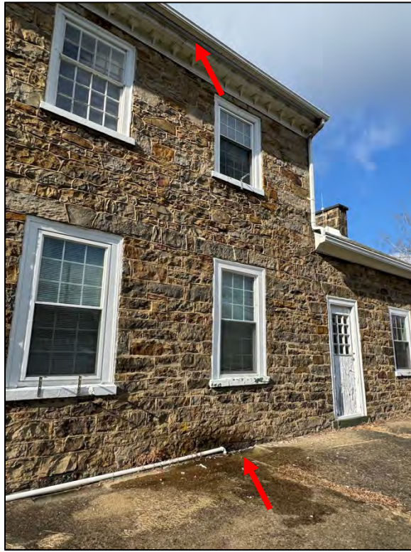
Plate 55. Image depicting the moisture directed to the foundation from faulty gutter.
