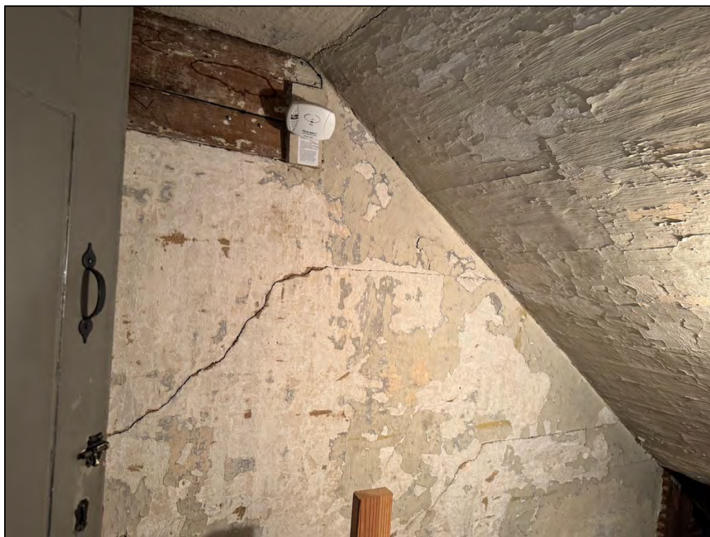
Plate 123. Room 1, basement entry, facing northwest. Note the crack in the plaster.
